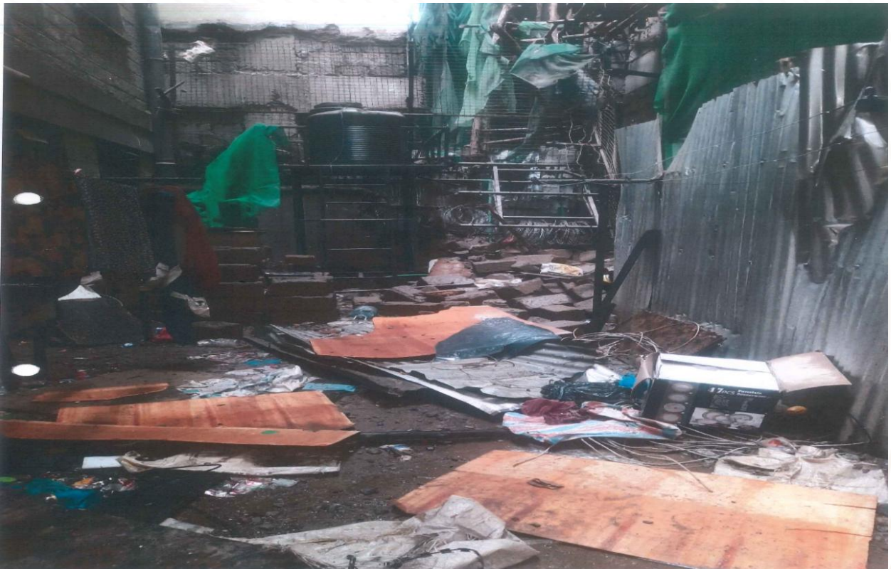
Figure 8: Pictorial Representation of construction materials/debris deposited on the backyard of Coldstone Limited property.
