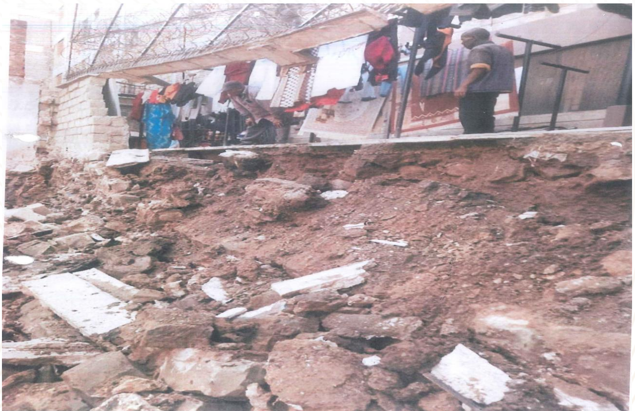
Figure 6: Pictorial representation of the demolished Boundary Wall belonging to Coldstone Limited.
